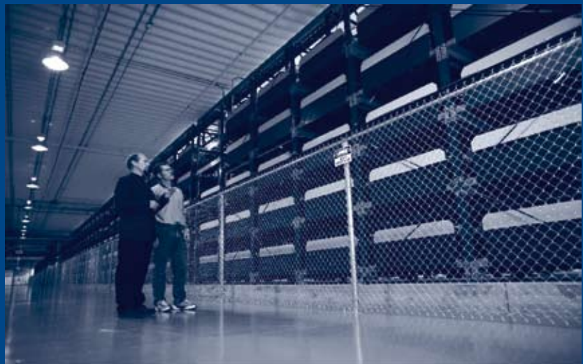
The world's largest Battery Energy Storage System (BESS Alaska) monitored with LEM current transducers
